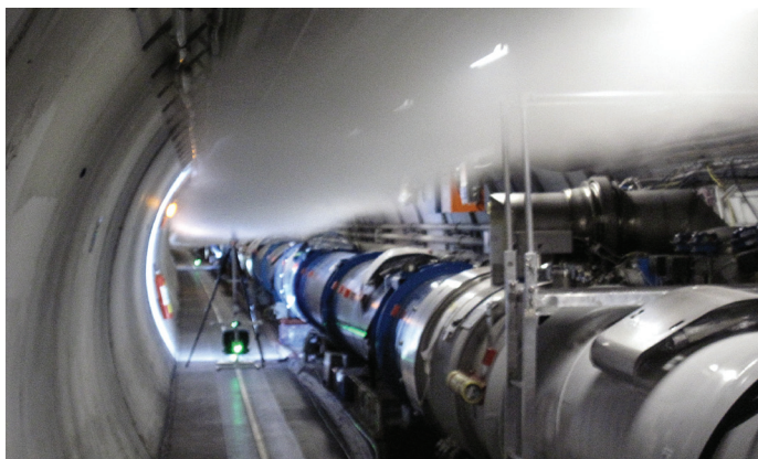
Three helium-leak tests were performed in the tunnel. (OPEN-PHO-SAFETY-2014-001)
