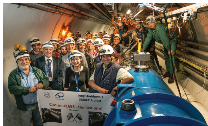
The final interconnection of the LHC superconducting magnets was closed on 18 June, after 14 months of work to reinforce the electrical interconnections. (CERN-PHOTO-201406-127 – 3)
