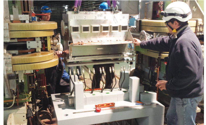
Installation of a FineMet cavity in the PS accelerator for the stabilisation of high-intensity beams. (OPEN-PHO-ACCEL-2016-003-5)
