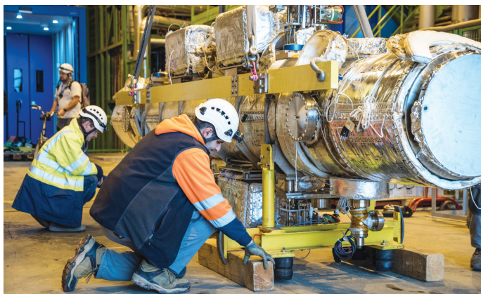
Preparation of one of the new beam absorbers for injection, installed during the year-end technical stop. (CERN-PHOTO-201601-004-8)
