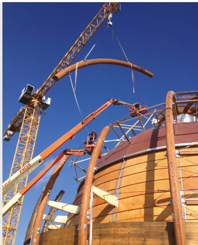
After 11 months of renovation work on the Globe of Science and Innovation, the Universe of Particles exhibition opened its doors again in April, and topped the TripAdvisor chart of tours and museums in the Geneva region. (BUL-PHO-VIEW-2015-002-7)
