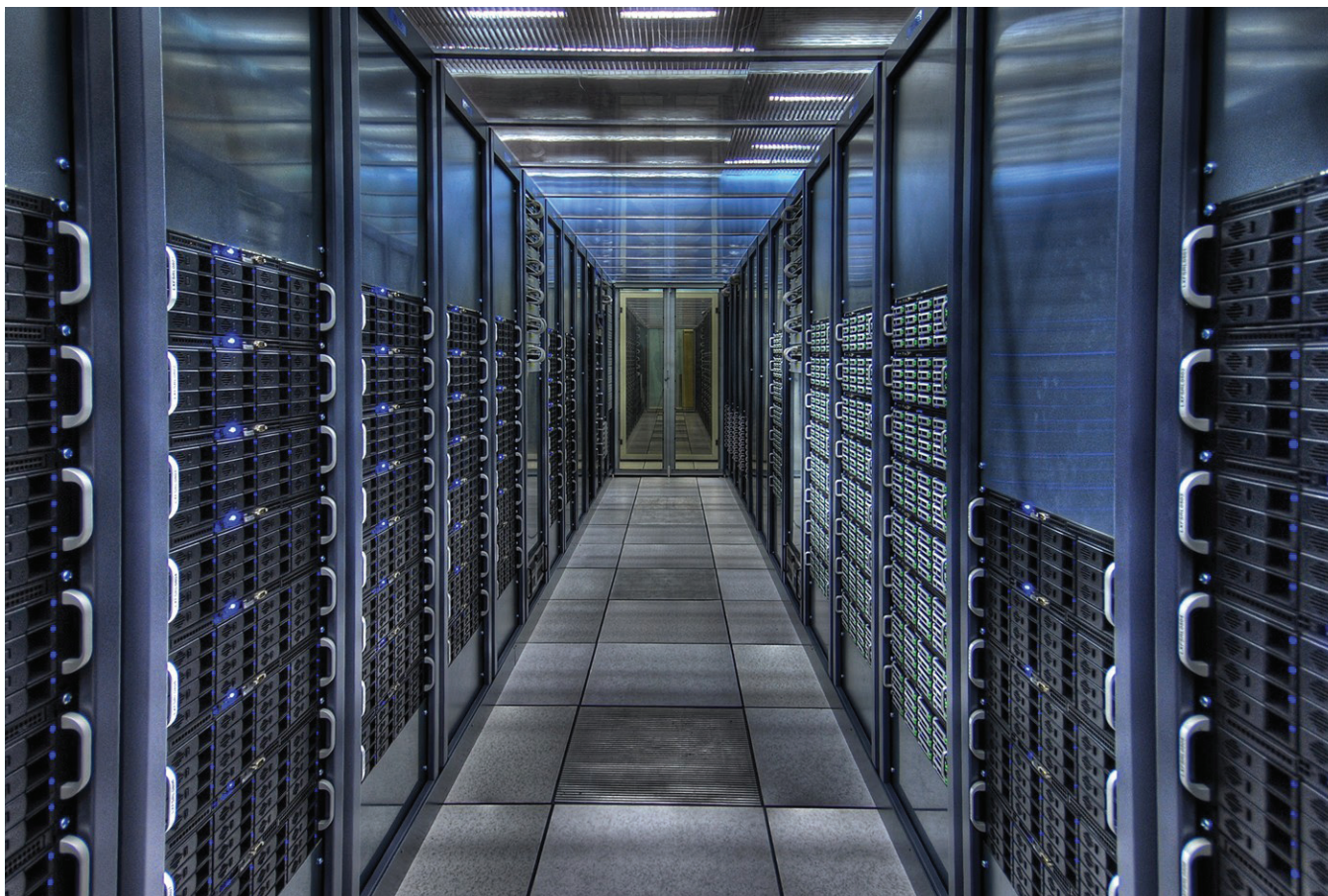
The CERN Data Centre houses servers, data-storage systems and networking equipment, not only for the Worldwide LHC Computing Grid, but also for systems critical to the everyday operations of CERN. (CERN-CO-1008289-04)
