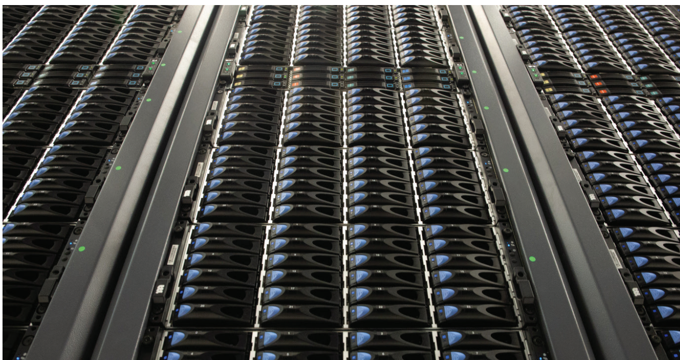
The CERN Data Centre houses servers, data-storage systems and networking equipment, not only for the Worldwide LHC Computing Grid, but also for systems critical to everyday operations at CERN. (IT-PHO-CCC-2018-001-13)
