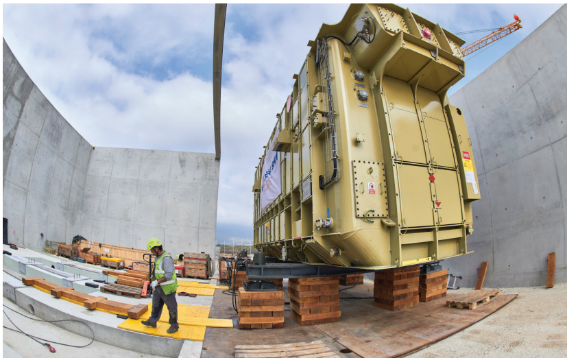
A new 400 kV power transformer, the largest at CERN, was delivered to reinforce the Laboratory's electrical infrastructure. (CERN-PHOTO-201810-254-31)
