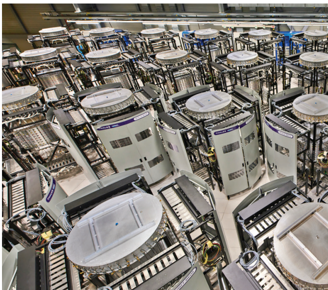
Installation of the new solid-state amplifier system developed for the SPS accelerating cavities. (CERN-PHOTO-201902-037-2)
