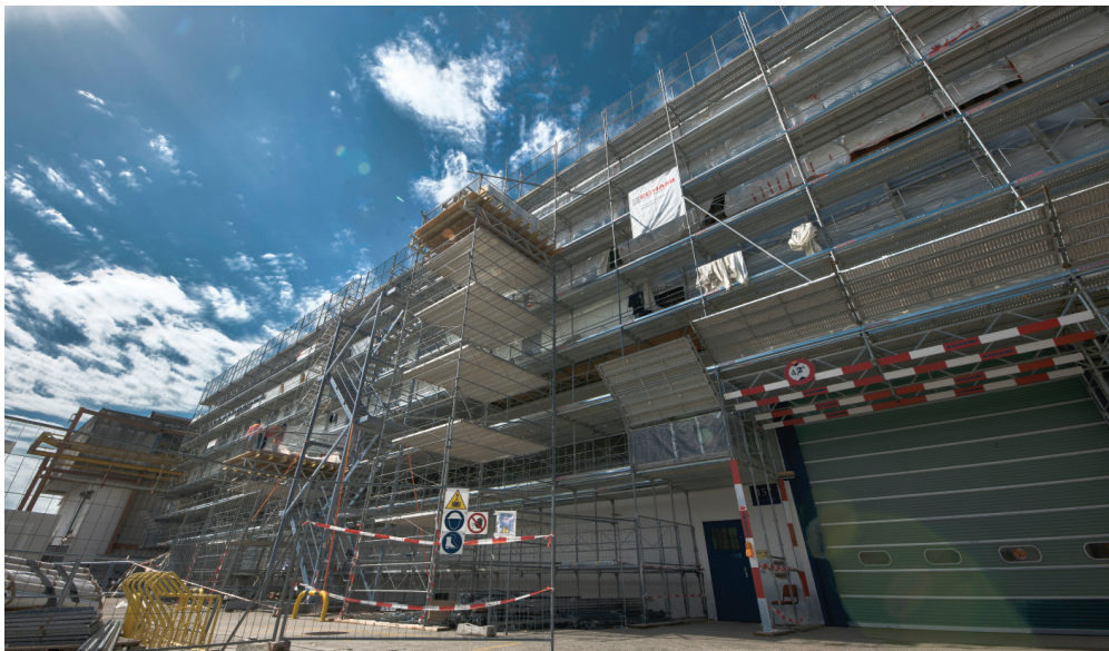
The new insulation installed on the huge East Area building will reduce thermal losses by 90%. (CERN-PHOTO-201805-130-3)
