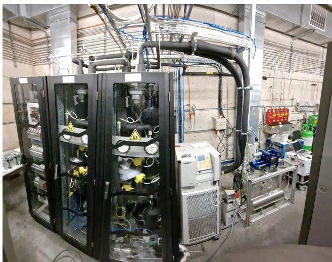
Picture of the first HFC-134a recovery plant for the specific RPC detector gas mixture. The plant was developed at CERN and has been operational at the CMS experiment since 2024.
