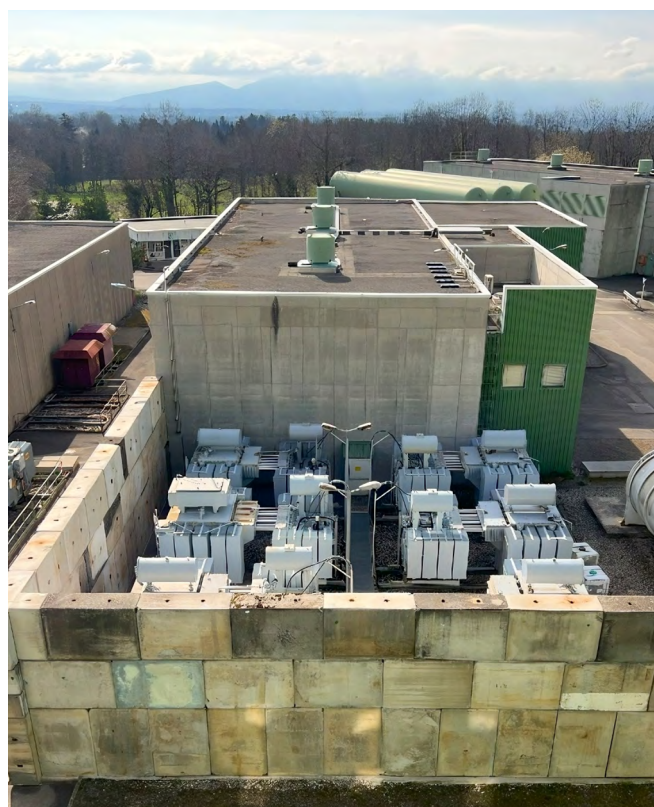
Acoustic barriers installed at LHC Point 4 (Échenevex, France) to reduce the noise impact of the electrical transformers.
