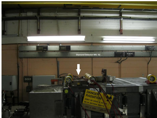
Figure 7: The white arrow in the picture indicates the position of the fast BLM on the top of main unit 42.
