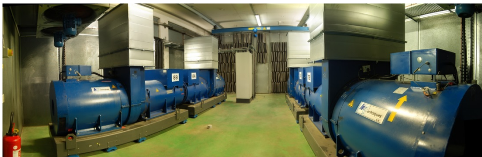
Fig. 31: Two twin rotablocs (four accumulators and four alternators in one cell)
