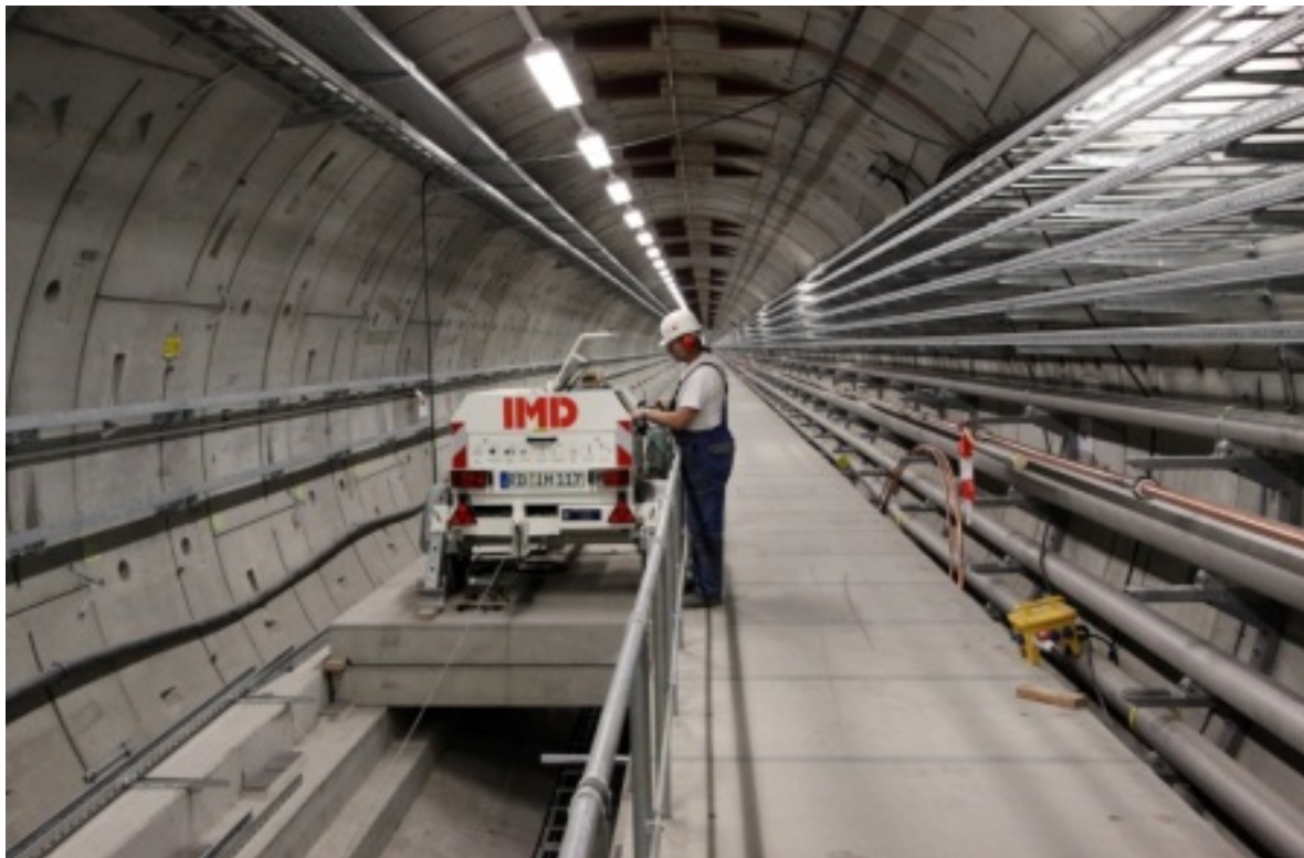
Fig. 7: The empty XTL tunnel at DESY Hamburg with the lights as the only heat sources
