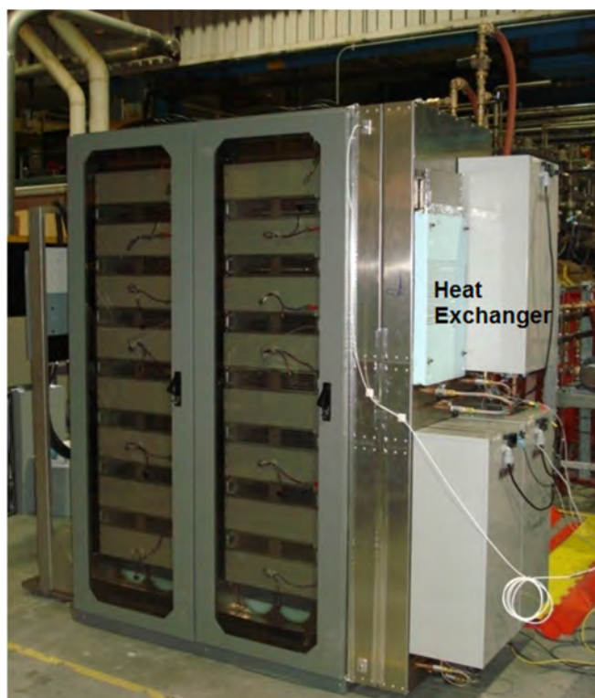
Fig. 8: NSLS-II sealed racks (equipment enclosures)
