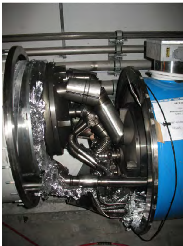
Fig. A.1: A damaged interconnect between a quadrupole and a dipole magnet
