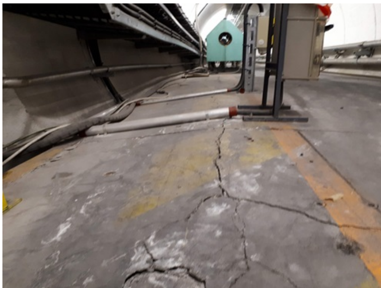
Figure 5.55: TT61 area of significant floor heave next to alcove.
