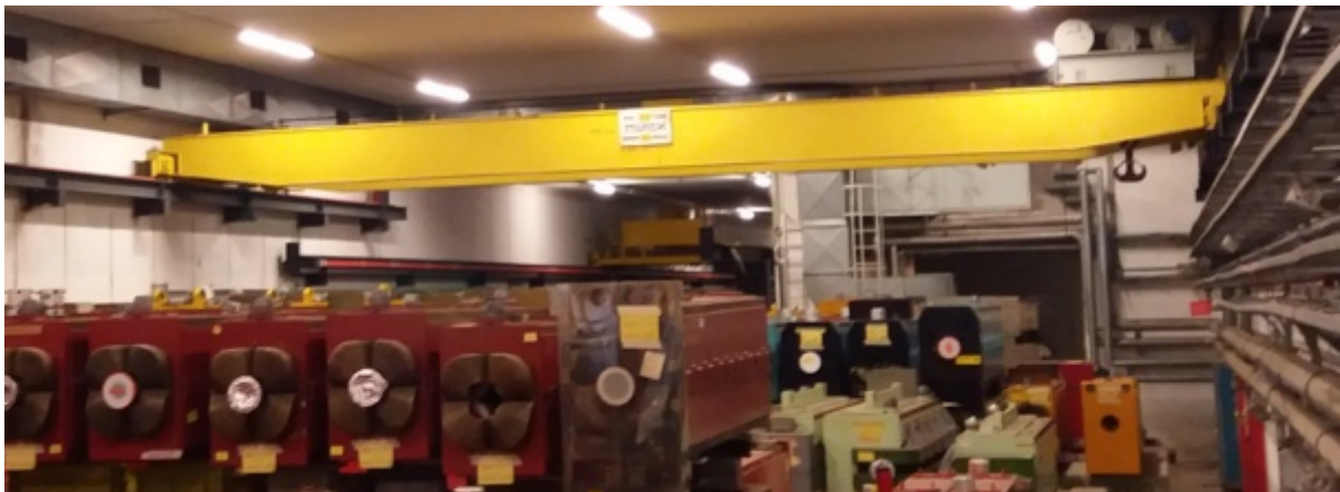
Figure 5.45: Current EOT crane in TT5.
