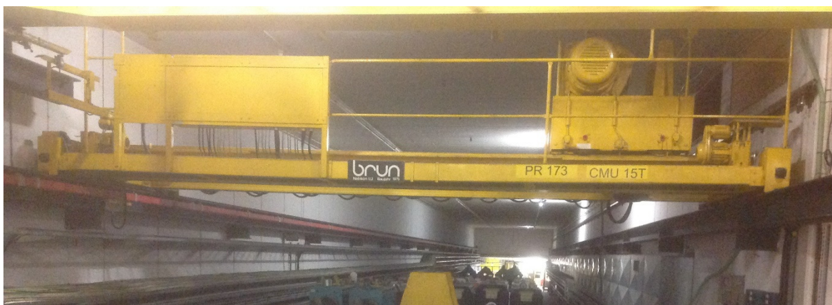
Figure 5.43: Current EOT crane installed in TT4.
