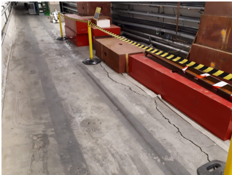
Figure 5.54: TT61 typical cracking in invert.
