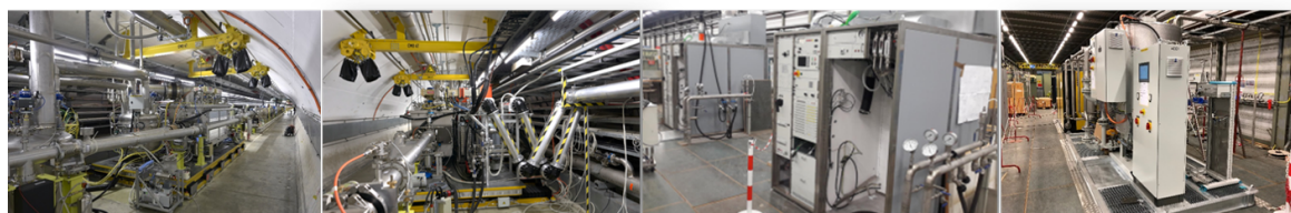
Figure 4.5: Surface and tunnel installation of the RF and cryogenic system in the SPS for crab cavity tests.
