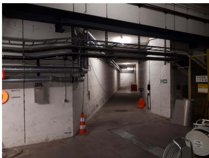
Figure 5.47: Access gallery TTA4 entering TT4.
