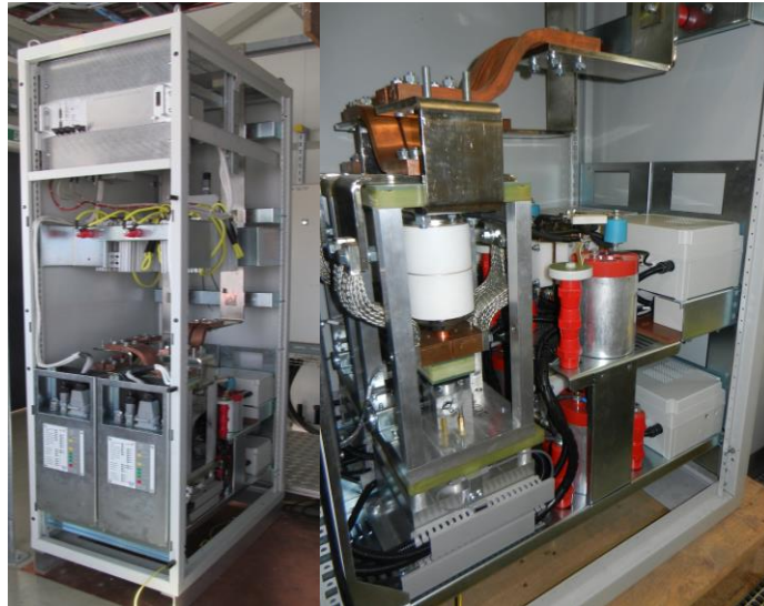
Figure 7-12: Prototype of 2 kA EE system based on vacuum breakers. Left: rack of first prototype; Right: Zoom on vacuum switch and auxiliary components
