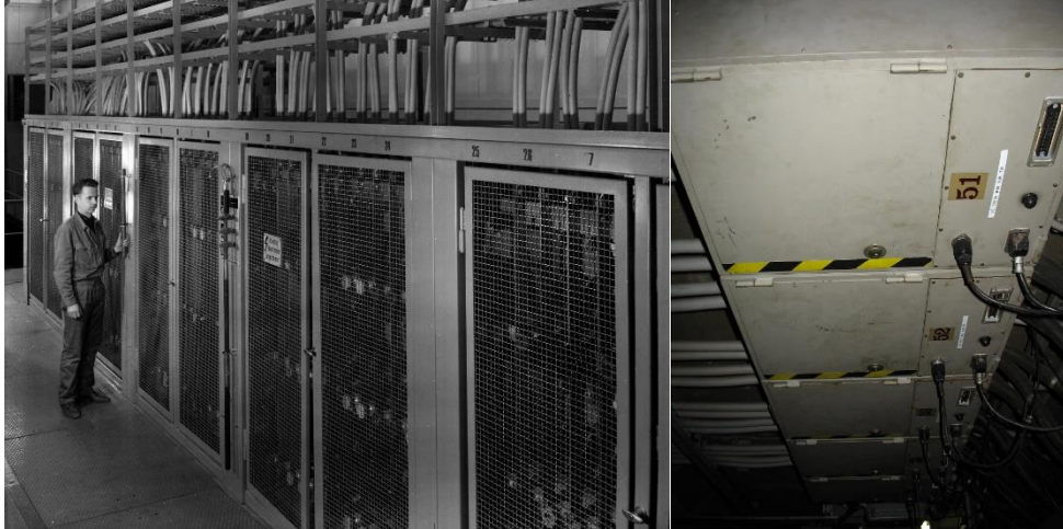
Fig. 5-15: Left: line selector in Building 251, right: terminal boxes in the technical gallery under Building 157.
