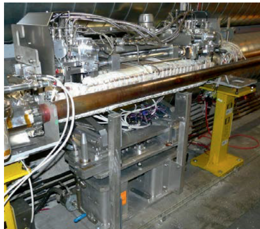
Figure 5-3: Photograph of the active absorber TCLA.B6R7.B1 as installed in the betatron cleaning insertion.
