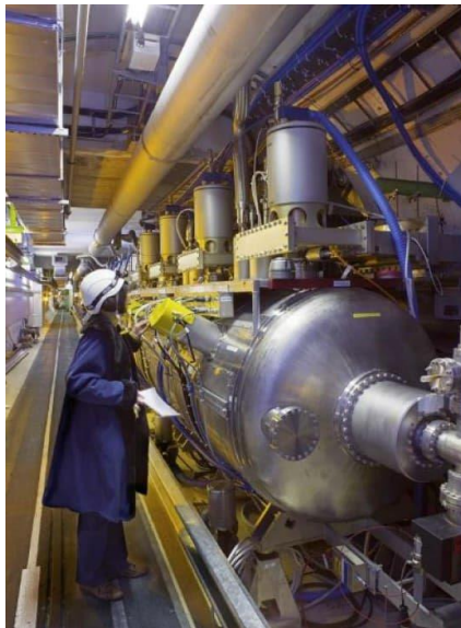
Fig. II.5.33: 400 MHz SC cavities in the LHC (former LEP) tunnel [25].
