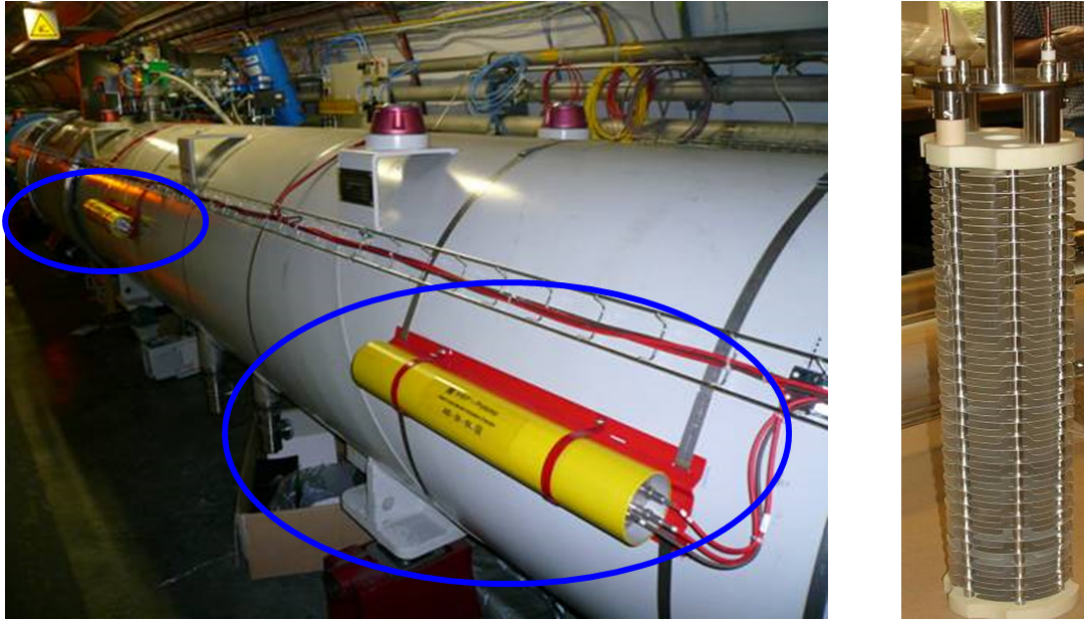
Fig. 19: Beam loss monitor at LHC
