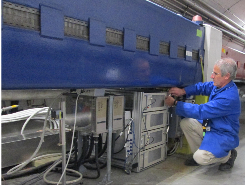
Figure 6: Photo of amplifiers in tunnel. 1 kW of 1 GHz bandwidth power amplifiers are available in this demonstration configuration to drive the beam. The amplifiers are located in the tunnel to minimize power loss in the cable plant
